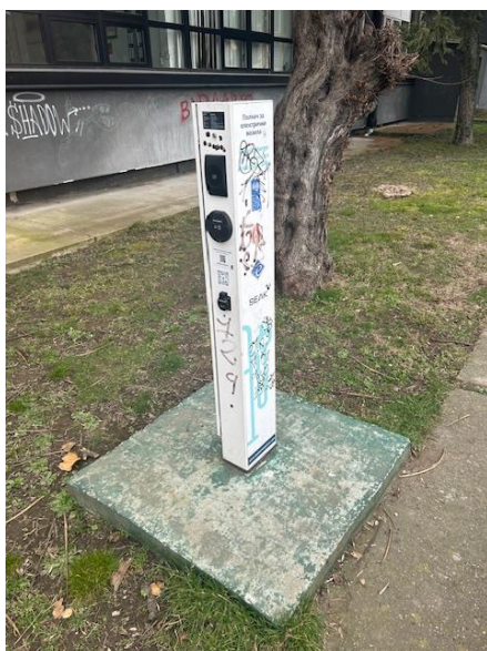
Fig. 6. INNOFEIT Living Lab 24 kW electrical vehicle charger
